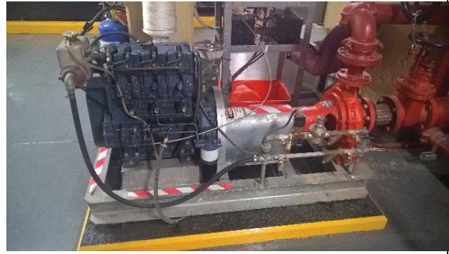
Photograph 4: A pump located within the basement plant room with fuel lines and oil filters observed and placed on bunding.
