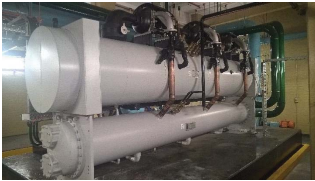
Photograph 7: Compressor / refrigerant unit observed on bunding within the basement plant room.
