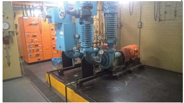
Photograph 8: Plant equipment installed on bunding and a drain within the basement floor.
