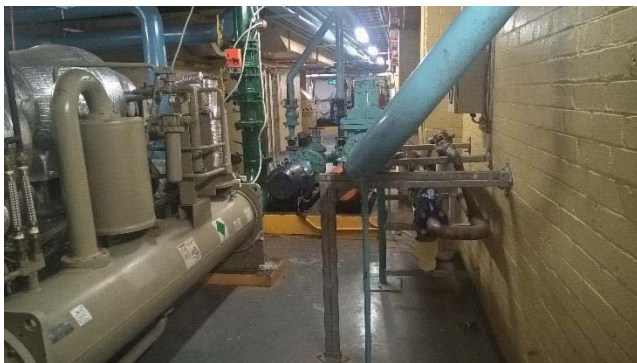
Photograph 5: Plant infrastructure located within the basement plant room.
